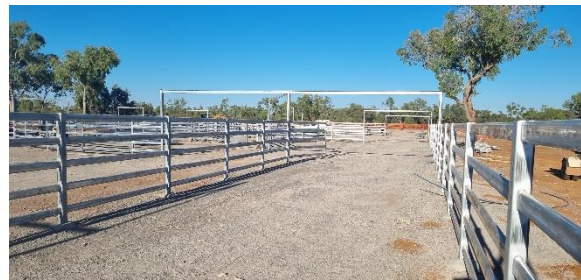
The new Cloncurry Saleyards Rail Load Out facility was completed in September 2024.
