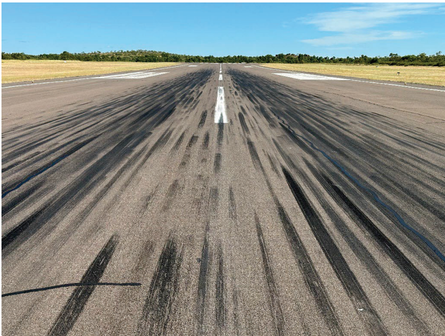
Photograph 8. Moderate rubber contamination in the Runway 12/30 touch down zone.
