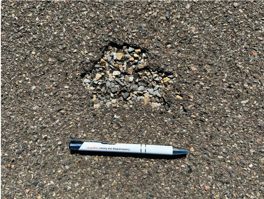
Photograph 3. Example of missing micro-surfacing from Runway 12/30 surface.
