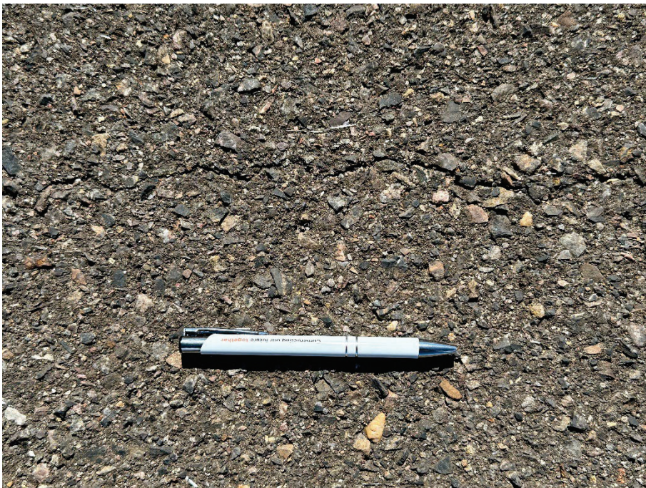
Photograph 4. Example of Runway 12/30 surface age cracking.
