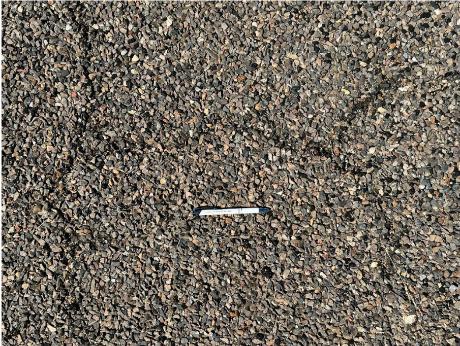
Photograph 15. Example of Runway 06/24 surface cracking.
