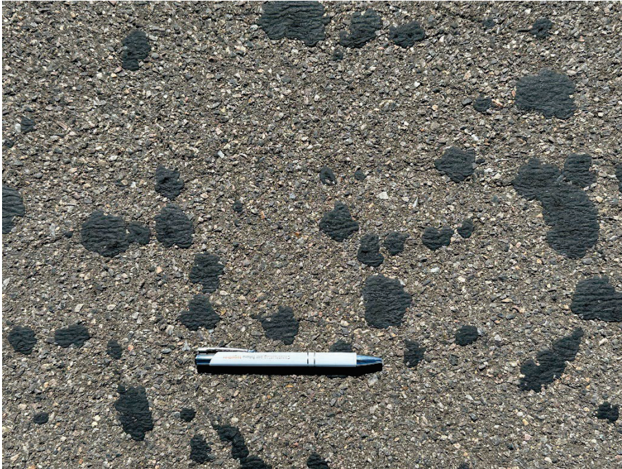
Photograph 5. Example of Runway 12/30 surface bleeding.
