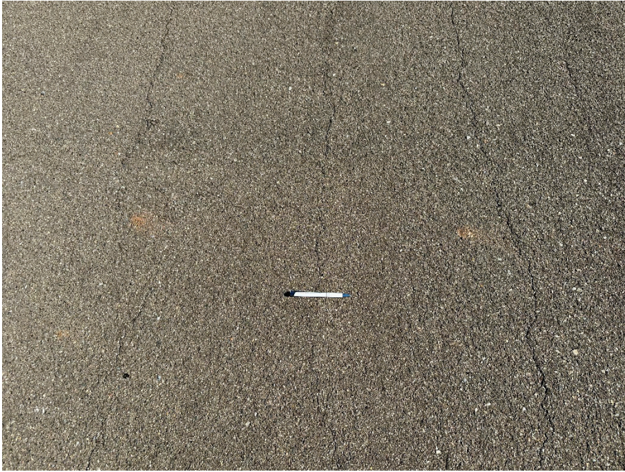
Photograph 7. Example of Runway 12/30 surface edge cracking.
