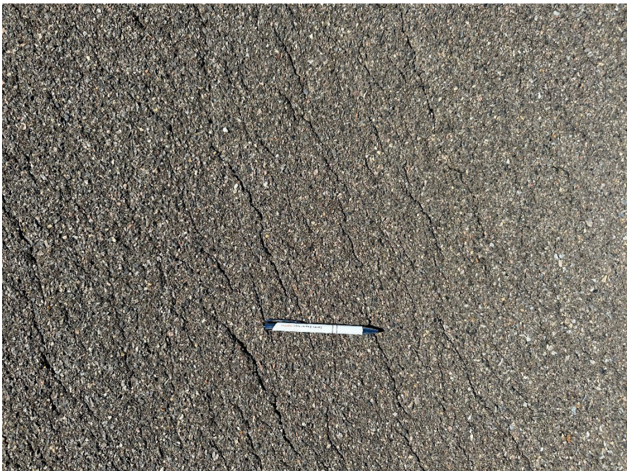
Photograph 6. Example of Runway 12/30 surface roller cracking.
