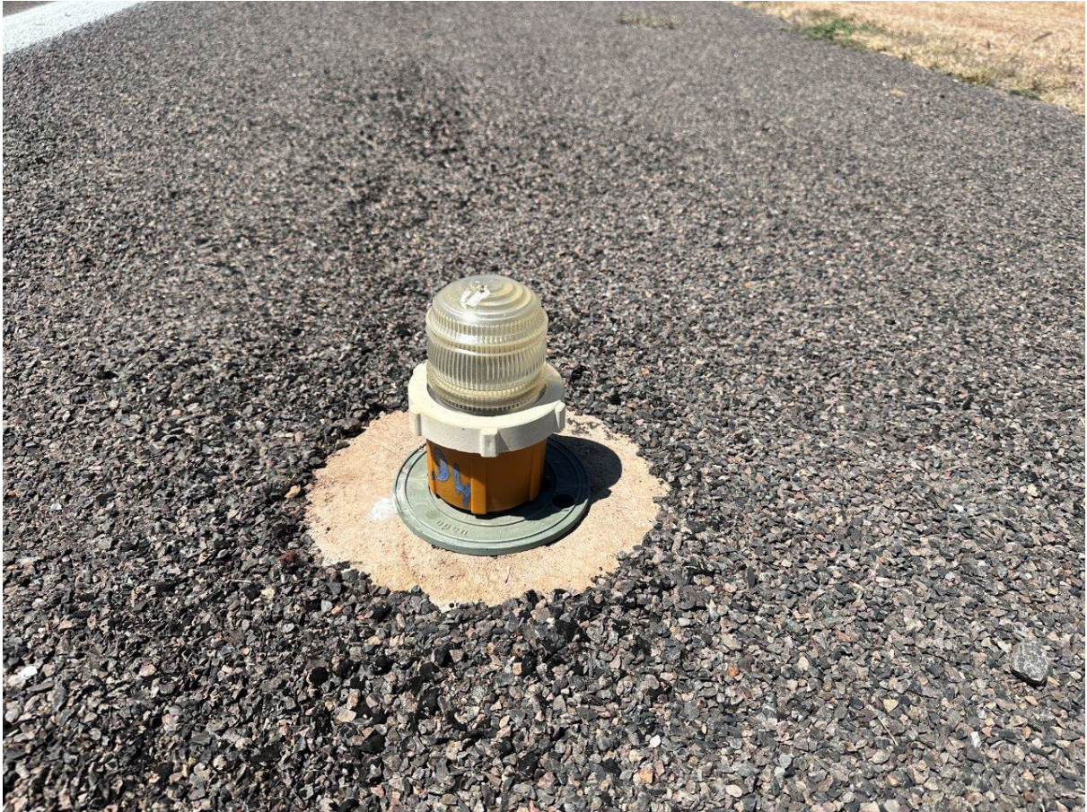
Elevated Runway Edge Light
