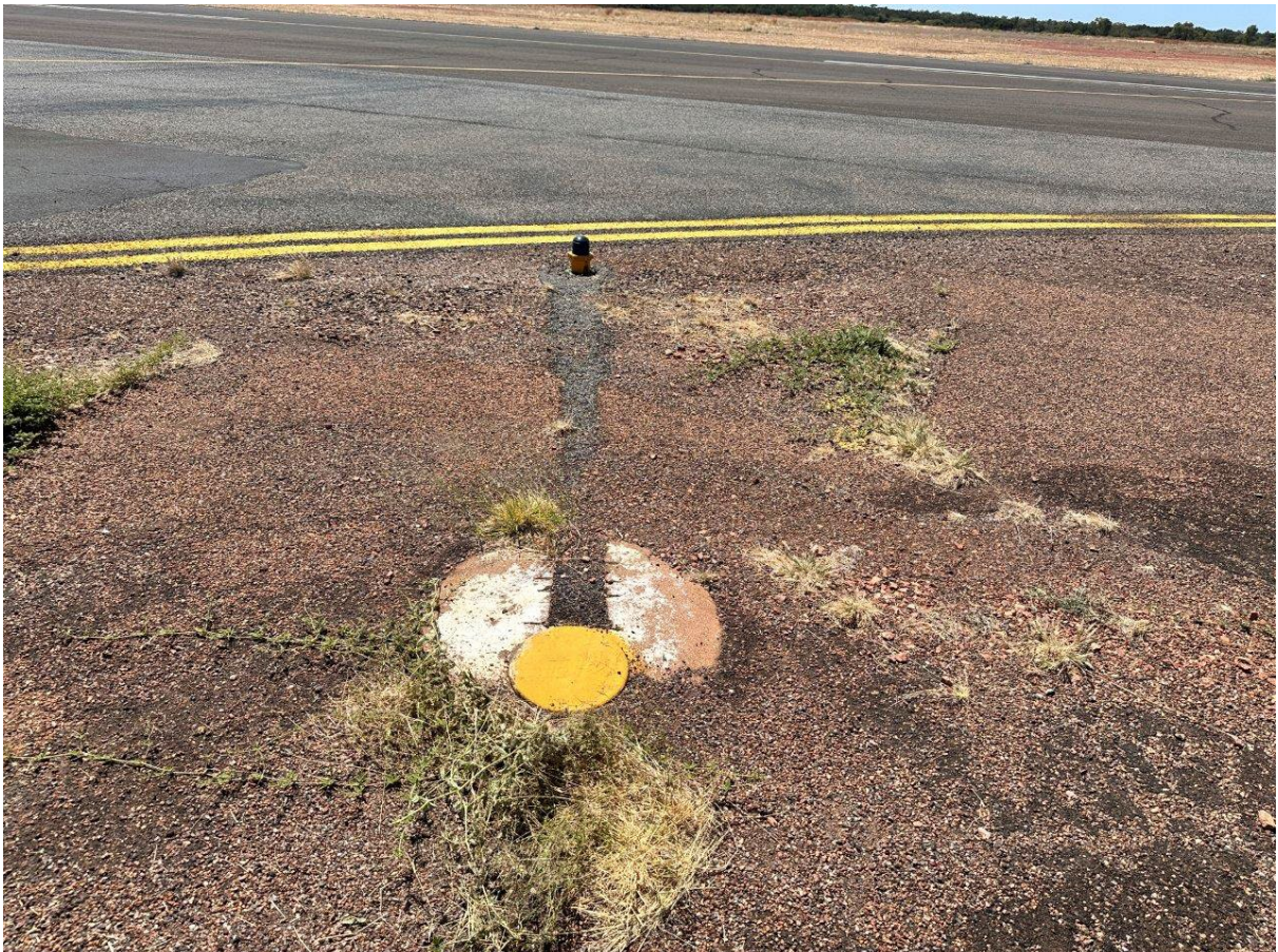
Taxiway B Edge Light
