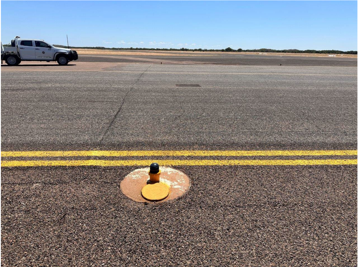
Taxiway B Edge Light
