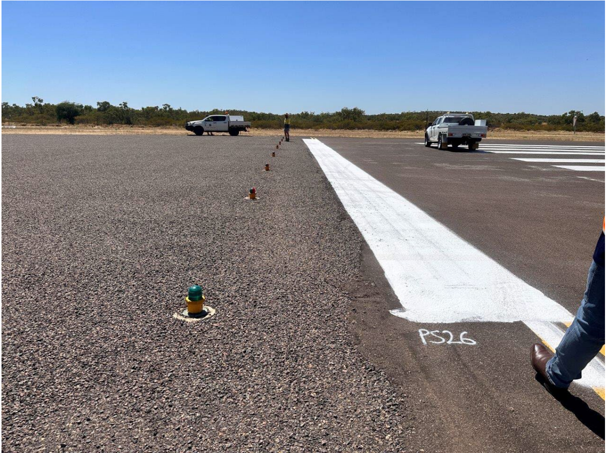
Outer Threshold and Threshold/End Lights
