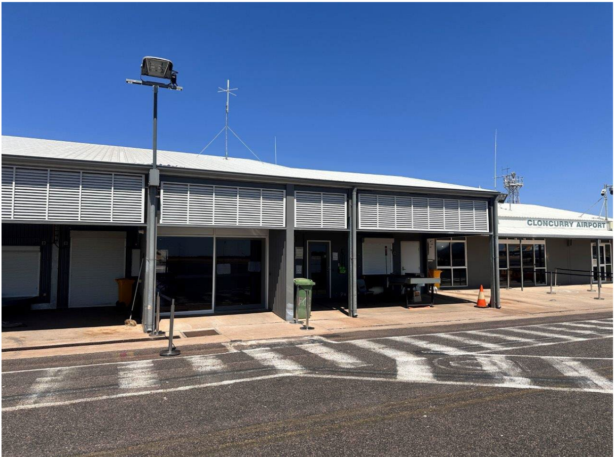
Apron Floodlight Poles (SW edge)
