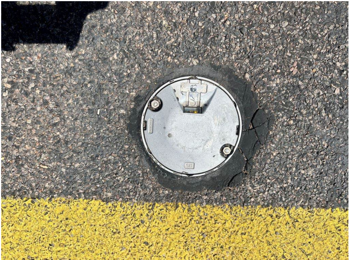
Taxiway A Centreline Light
