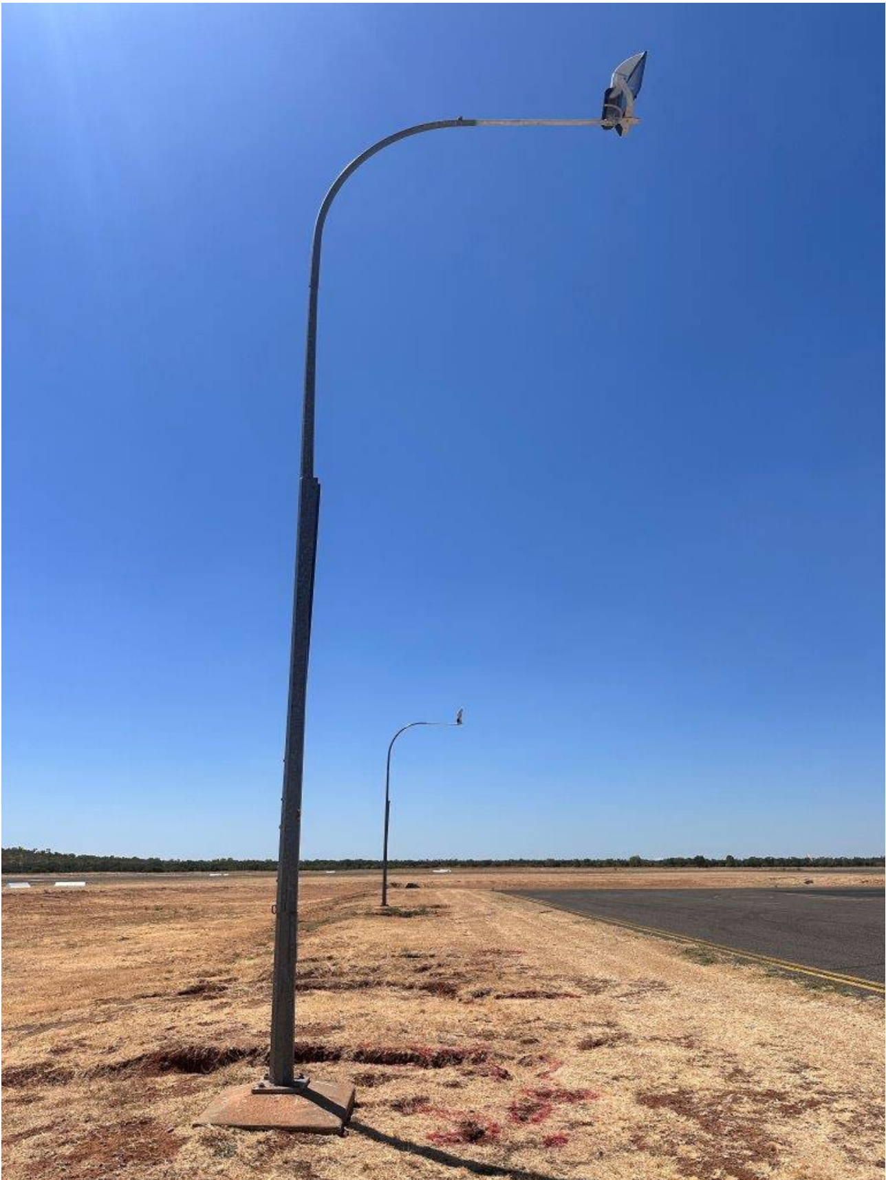
Apron Floodlight Poles (NW edge)
