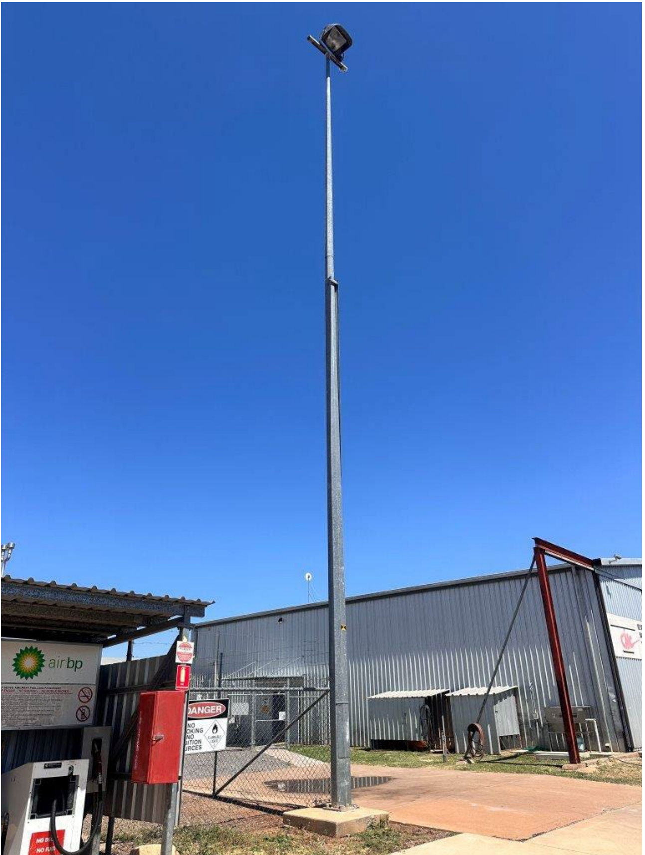
Apron Floodlight Pole (SW edge)
