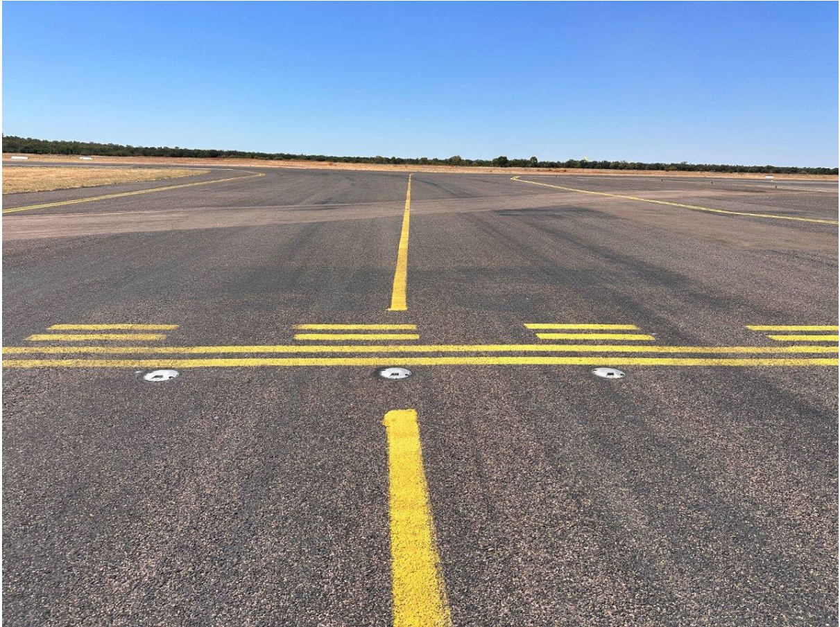
Taxiway A Holding Position Centreline Lights
